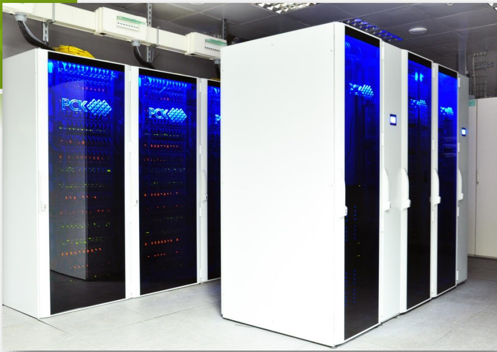
TORNADO SUSU COMPUTING CLUSTER
