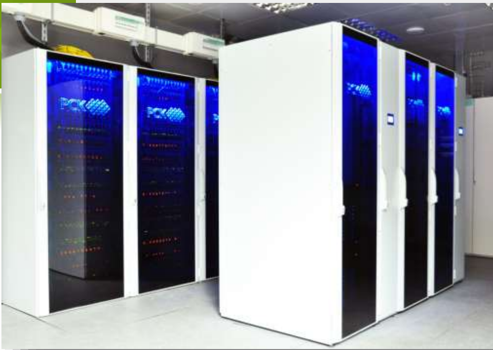
TORNADO SUSU COMPUTING CLUSTER
